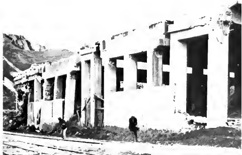
Photo 3. Damaged San Fernando Road overhead [2].
